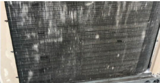
15 year old 5-ton roof unit before cleaning and coating
